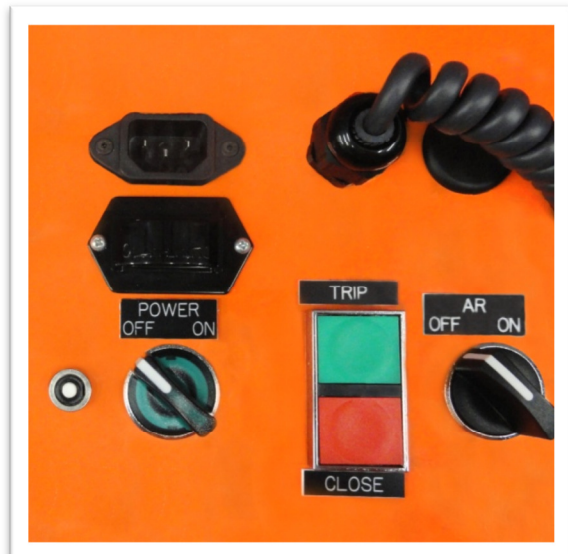
Figure 7: RSO-I control panel
