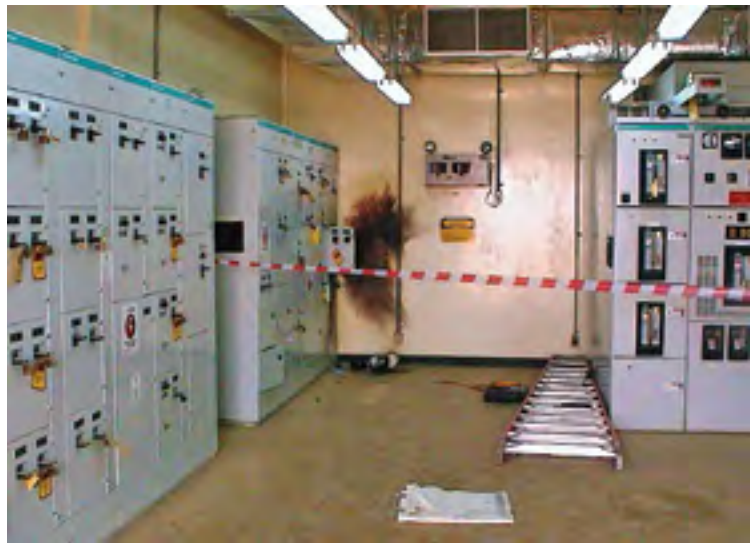
March 4, 2009, at the Jubail Project in Riyadh, Saudi Arabia. Three workers were removing a 480-V, molded-case circuit breaker from the bucket of an energized motor-control center (MCC) when an electrical arc flash occurred, severely injuring them. All three sustained first- and second-degree burns and were hospitalized following the accident. Myth: Switchgear is designed with arc-flash containment in mind.
