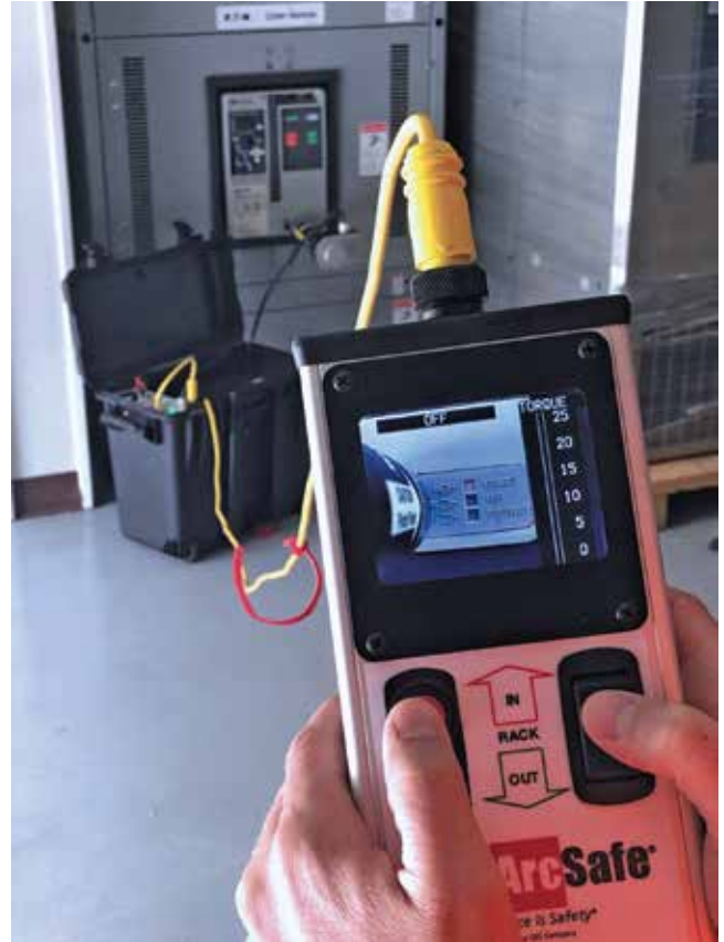
Video-enabled controller with camera for watching the Magnum DS position indicator. On the right side of the screen is the torque bar graph monitor.
